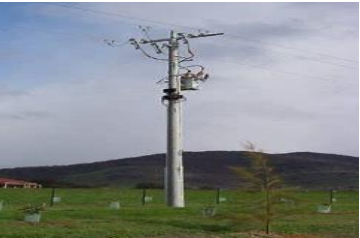
Power Distribution Poles
