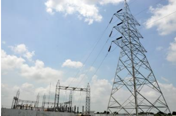
Transmission Line EPC
