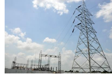
Transmission Line EPC
