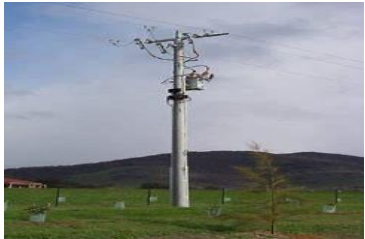
Power Distribution Poles
