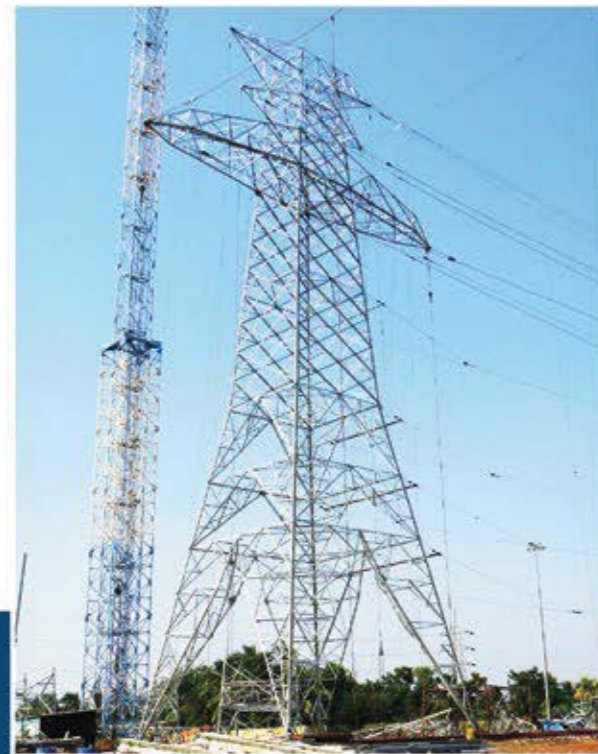
500kV HVDC Egypt
