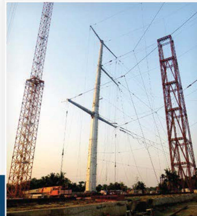
765kV S/C Monopole for India
