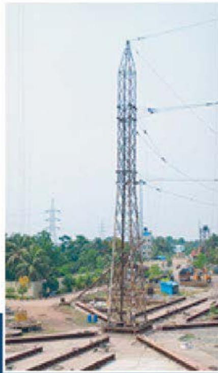
220kV Substation Column India
