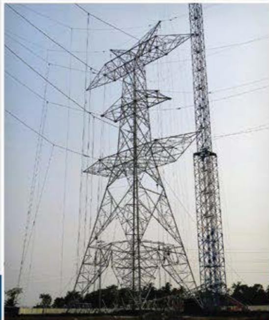
400kV DC Twin TL
