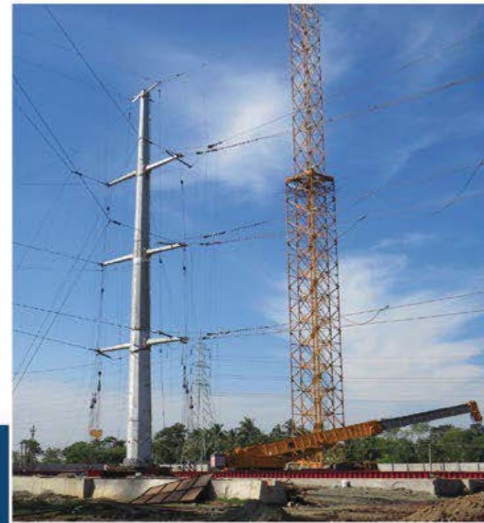
400kV D/C Quad Moose Monopole
